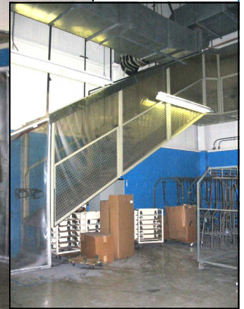
Fully enclosed clean tunnel enclosing painted parts going to oven.
