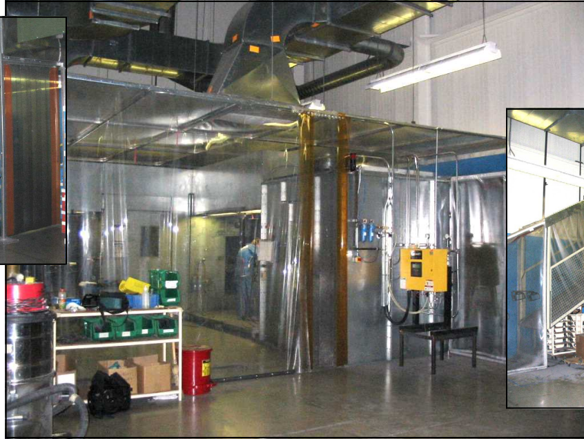
From parts wash/blow-off to paint booth enclosed within one positive pressure clean air environment.
