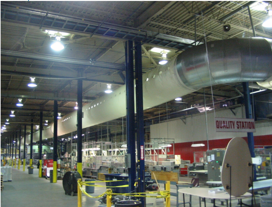
The fabric ducts were attached to metal elbow corners
